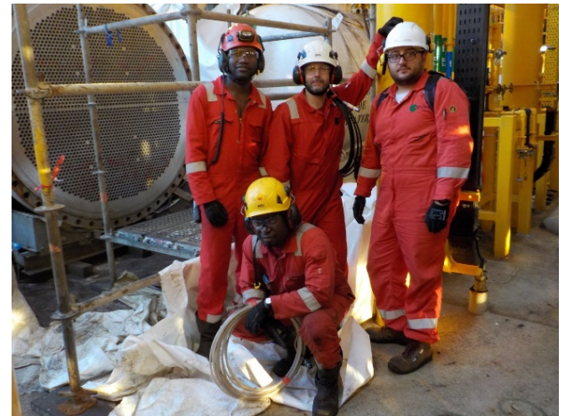
TOTAL E&P Angola, FPSO "CLOV" – Tube Inspection
