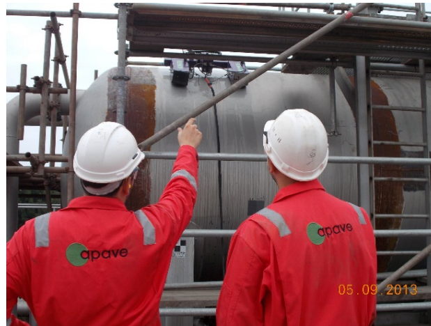
SHELL, Gabon - Vessel Corrosion Mapping using RMS and UT
