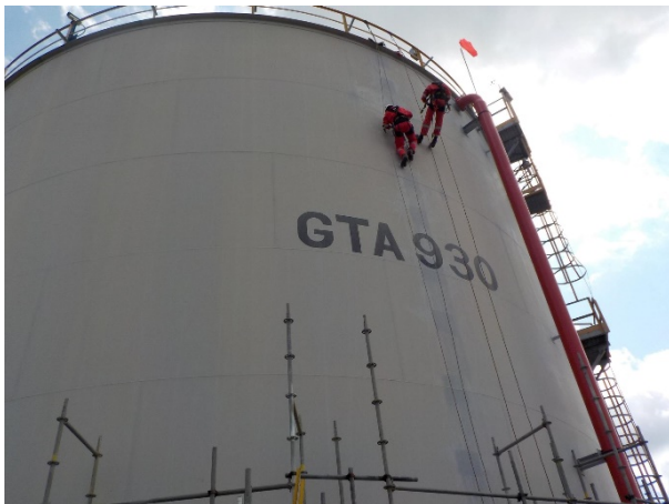
TEPB, Brunei - Scanning Storage Tank dents using 3D Laser camera - Creaform
