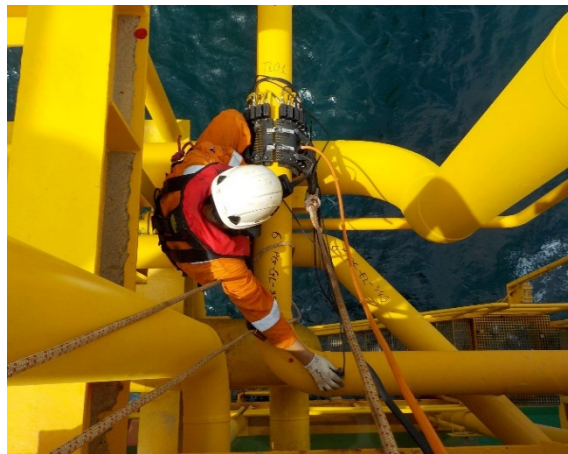
JVPC, Vietnam - Rope Access - LRUT and UTM from 3" to 16" pipes - CPC RANG DONG Platform
