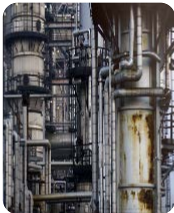
RBI and Integrity Assessment
