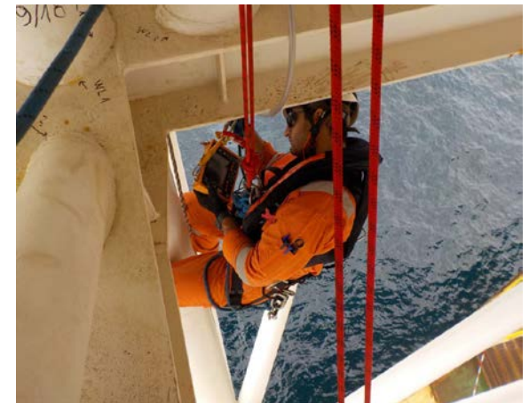
MODEC, Ghana - Rope Access - Eddy Current on Welds, Helideck Structure Fatigue Critical Joint - KWAME NKRUMAH FPSO M21
