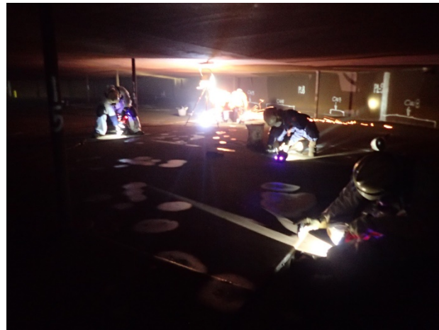
Marathon Oil, EG - Visual and MPI inspection after pitting repair - Storage tanks
